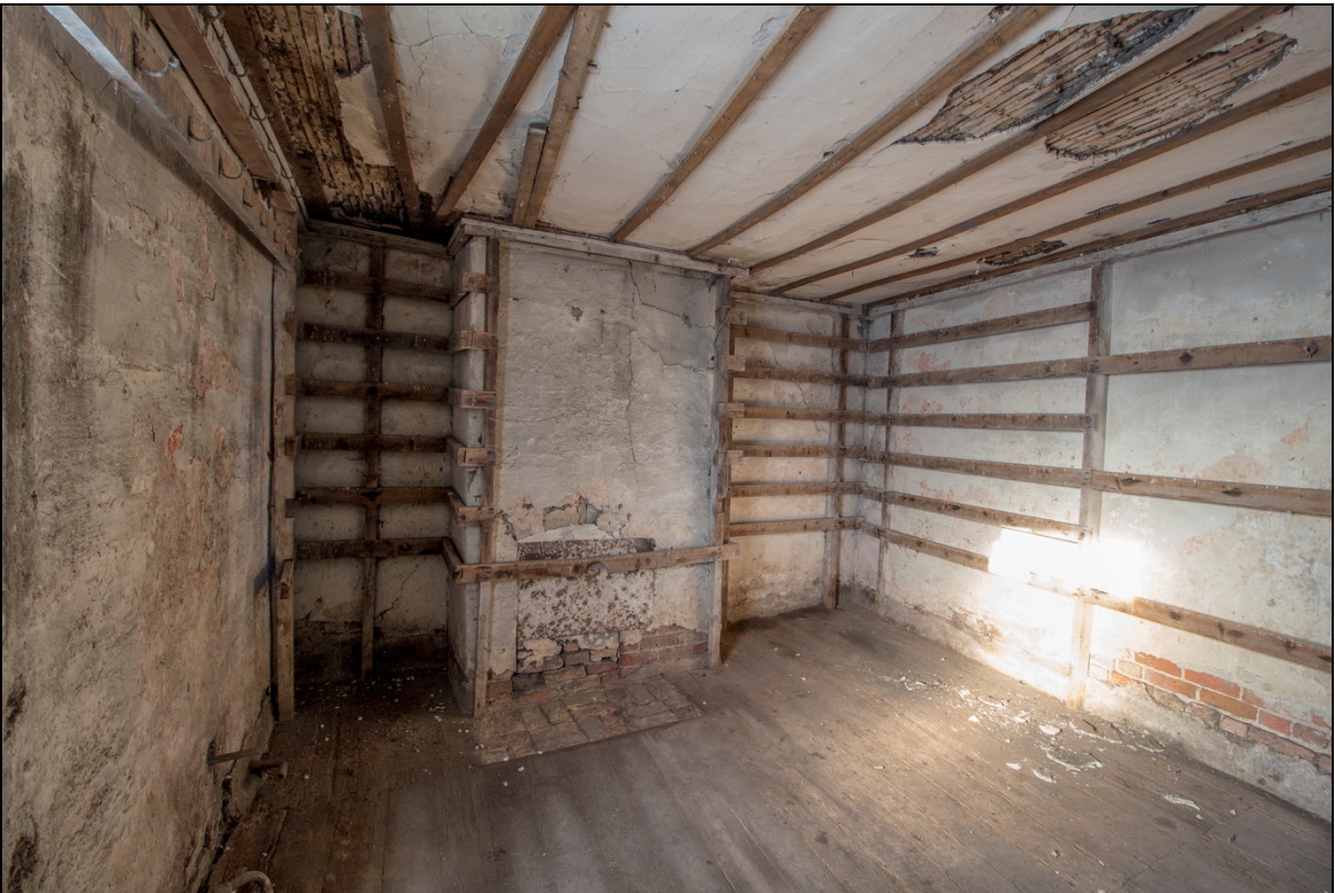
Second floor room where significant cracking is evident on party wall with 2 Nene Quay
