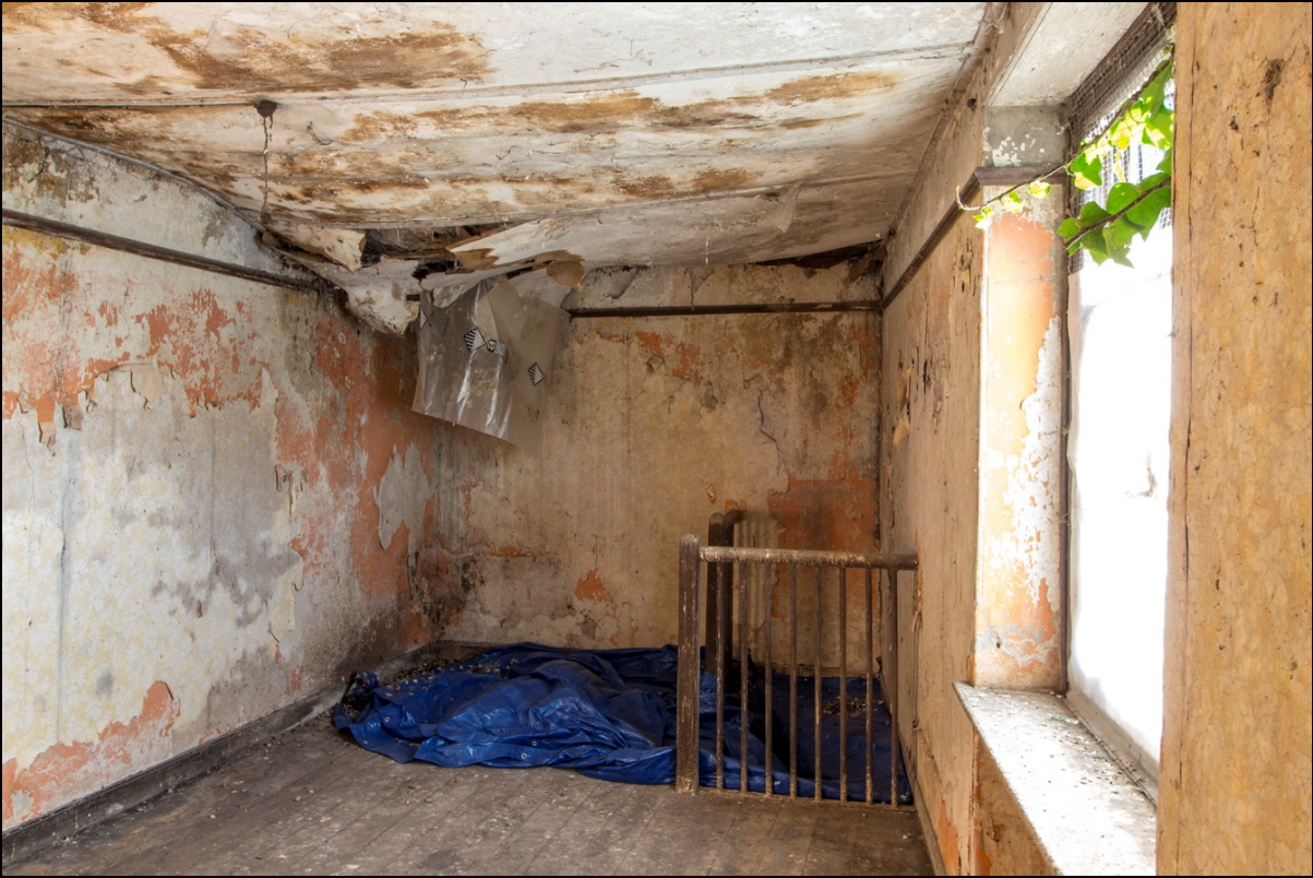
Damage to ceiling caused by 2 nd gap in roof covering
